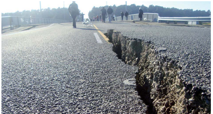
■ The Christchurch earthquakes cause damage and destruction.
