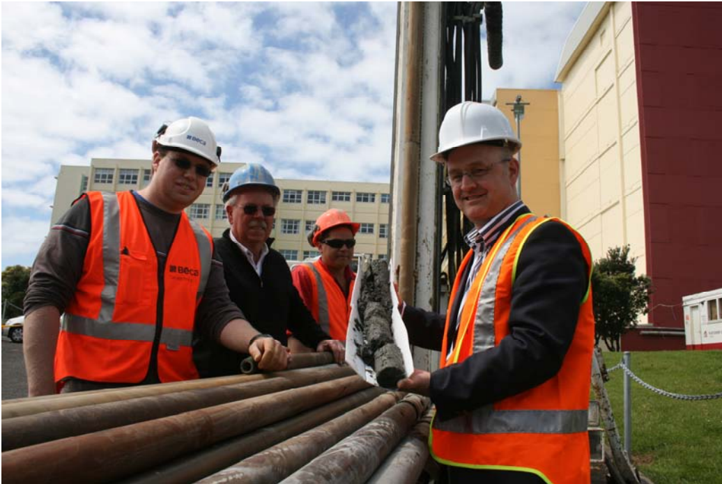
TDHB Project Coordinator Russell Hughes (second from left) and Tony Foulkes (right) with Pro Drill representatives.
