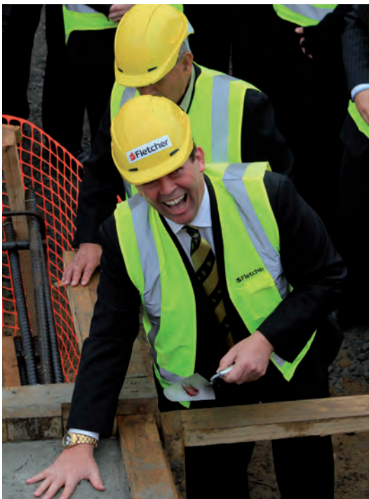
Above: MP Jonathon Young sets his hand print in the foundations of the new build.
